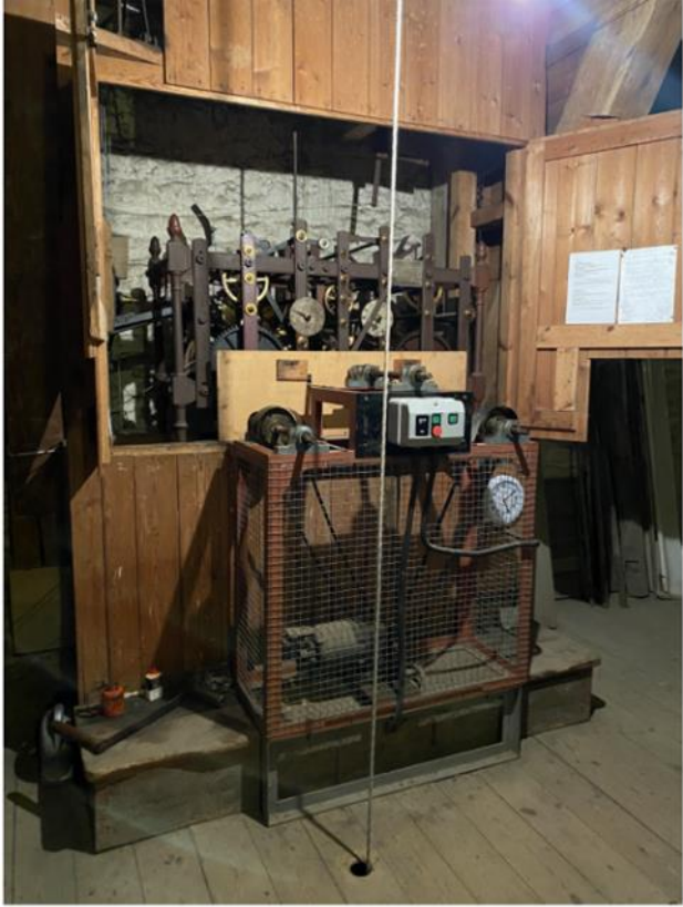
View of clock cabinet with electric winding assist installation in front. Photo: Rupert Griffin
